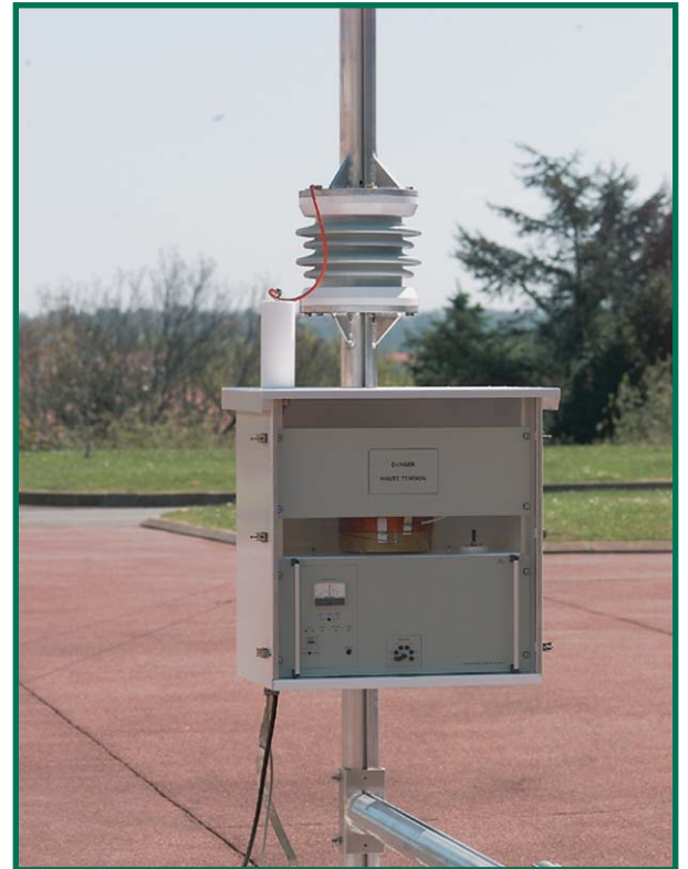
DAA 9400 I ON THE FOOT MAST OF THE UMBRELLA ANTENNA
