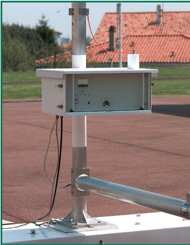
UAA 9400 I ON THE FOOT MAST OF THE DAISY ANTENNA
